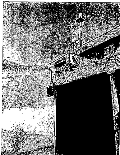
A. "All-in-one" installation with radar, solar panel, and telemetry unit mounted on side of bridge
